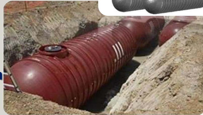
Underground Storage Tank System
