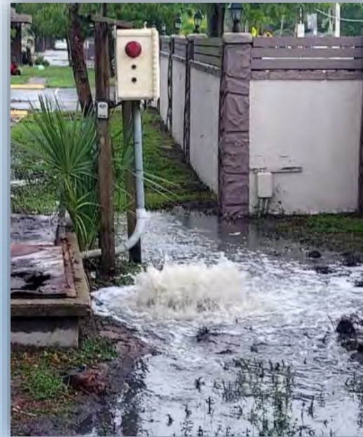
Private sewage pump station overflow
